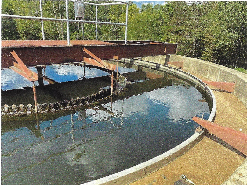
Figure 3- Clarifier in use at site visit
