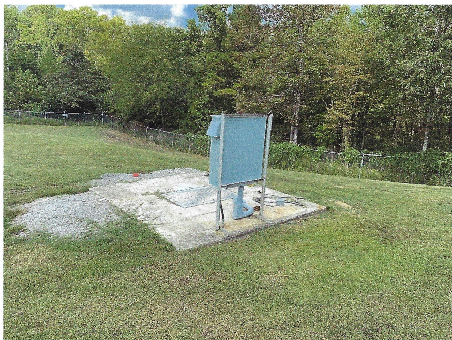
Figure 4 - New RAS Station
