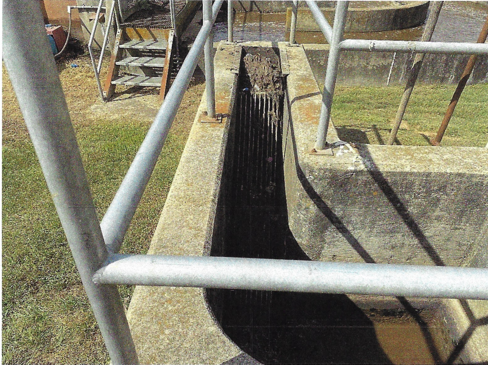
Figure 1- Head works bar screen
